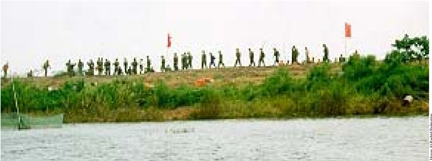
All hands on deck: since the founding of the People's Republic of China mammoth engineering projects have been built, including nearly 250,000 km of flood prevention/control dykes, 84,000 reservoirs of all sizes, 12,000 km of tide barrage and more than 490,000 irrigation and drainage stations.
