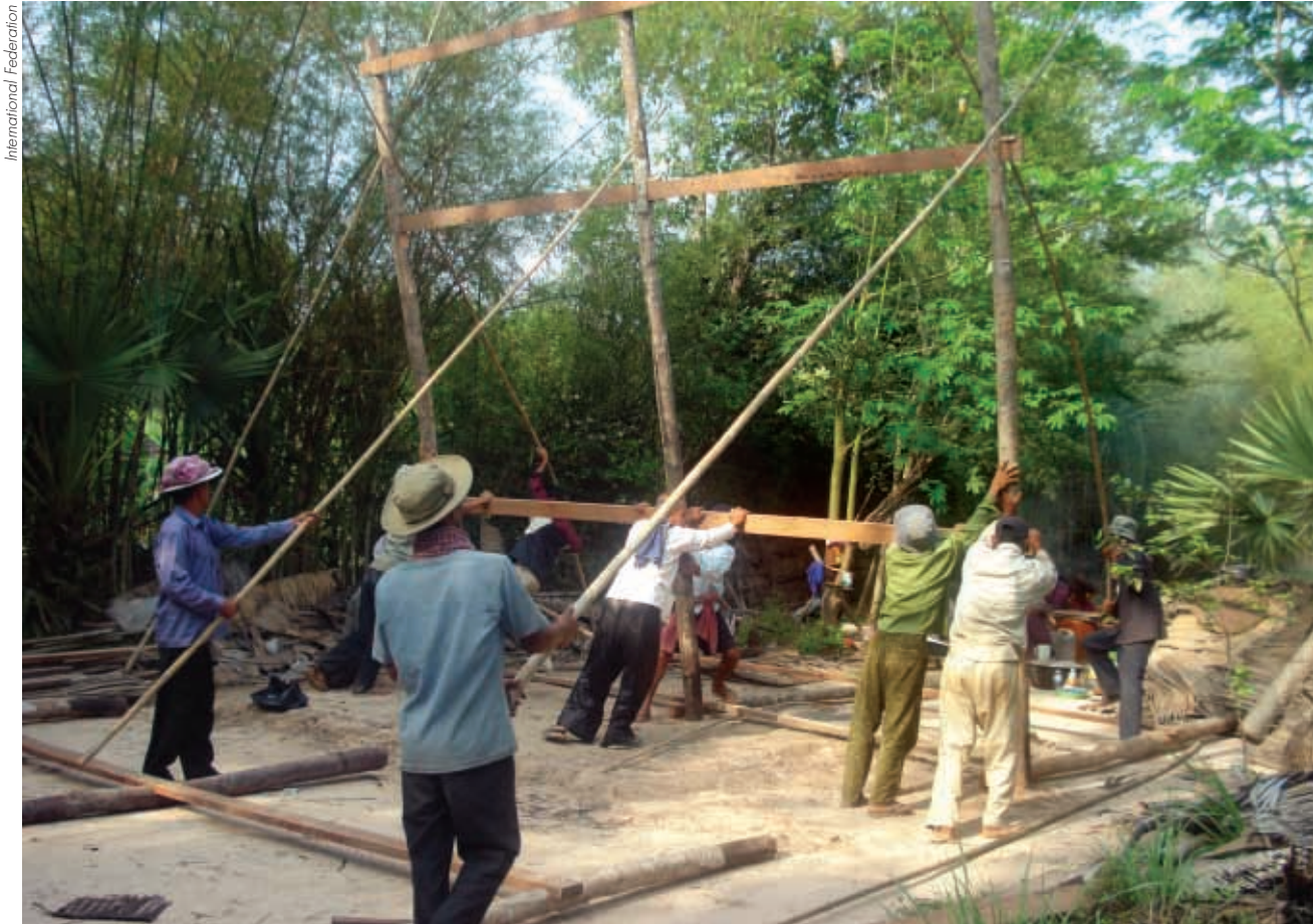
Beneficiaries collaborating on a housing project – disaster risk reduction measures in China.
