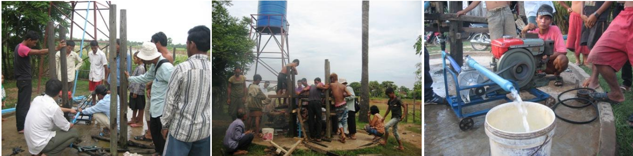
Villagers actively involved in installing water tank in their village. Photo: CRC/DMD
