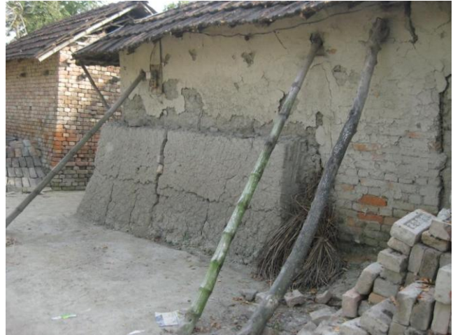
Prolonged water logging caused the plinths and walls of the houses to disintegrate and be near to collapse. Photo: IFRC.
