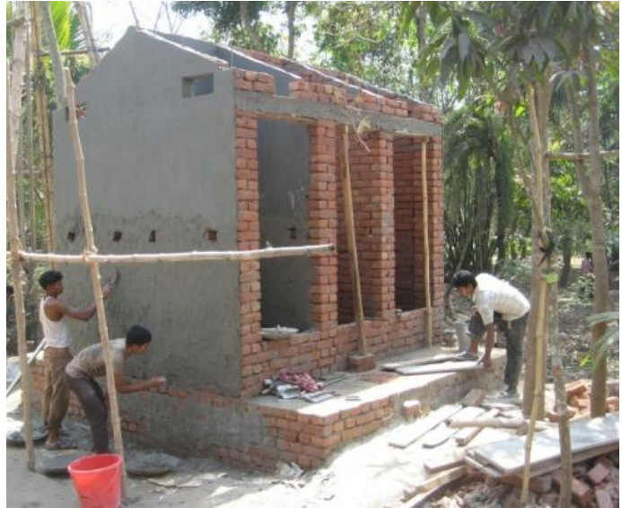
Construction of community latrine in location two of Jessore district. Photo: IFRC.
