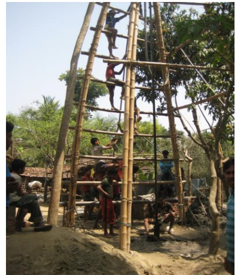
Community people involved in water pump installation near a community latrine supported by BDRCS Federation in Jessore district. Photo: IFRC.
