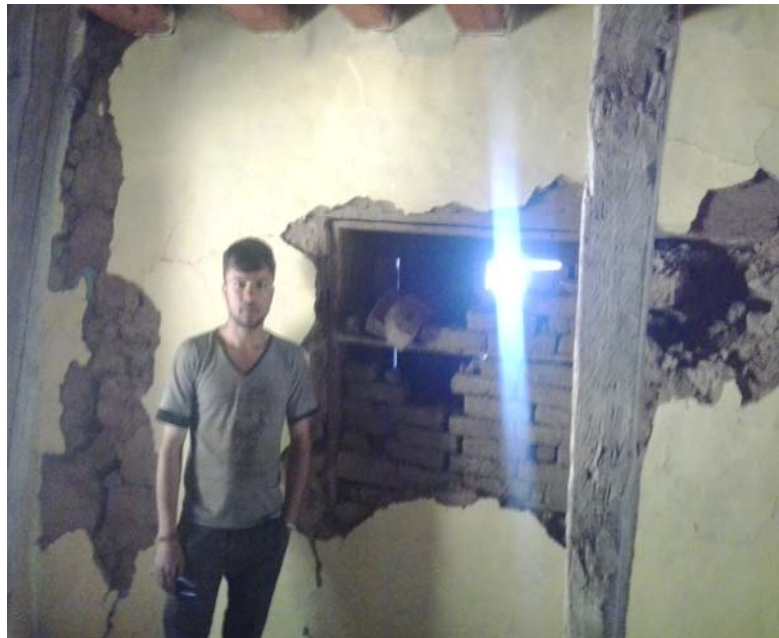
Inside one of the many damaged houses in Basthi Koti, Doda. Photo: Indian Red Cross Society.
