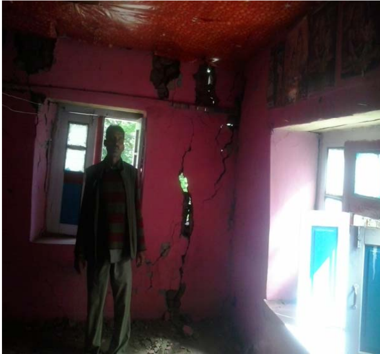
A damaged house in Banigra, Doda. Photo: Indian Red Cross Society.
