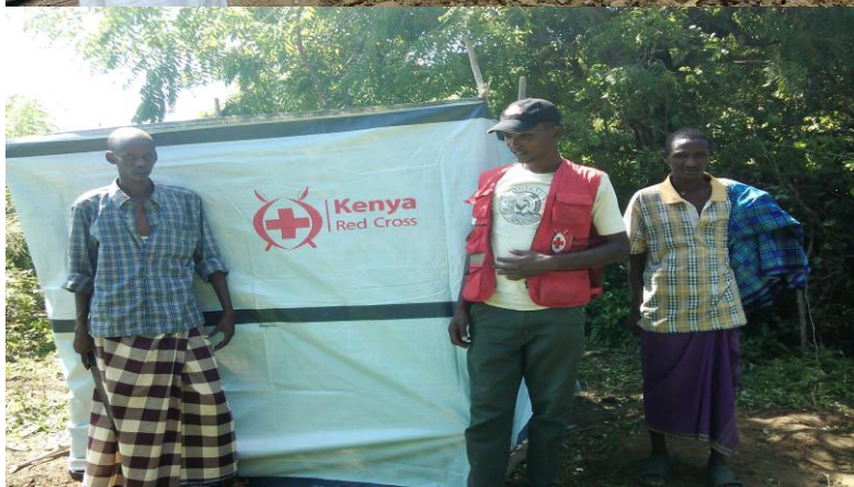
KRCS volunteers work with IDPs to construct latrines at Umoja IDP camp in the Coast region. A completed latrine. Photo/KRCS
