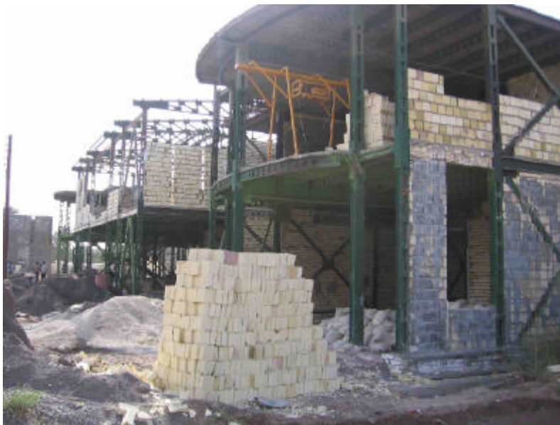
The construction of the Kafi school was accelerated, enabling to move on to the next phase of implementation
