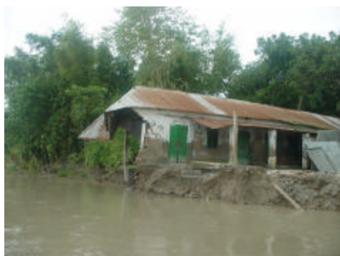
House damaged by floods in Sirajganj
