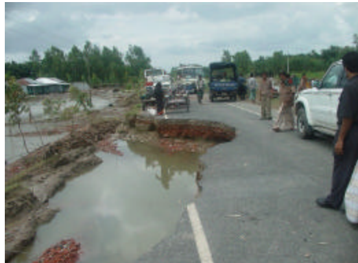
There has been heavy damage to infrastructure and roads throughout much of Bangladesh.
