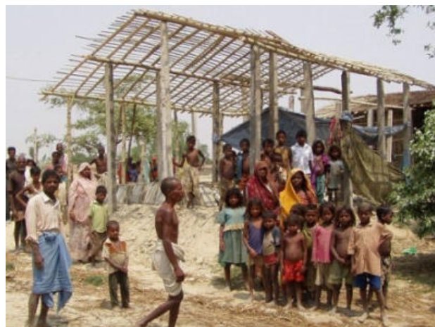
Part of the rehabilitation activities conducted by the Nepal Red Cross is the construction of houses for affected families.
