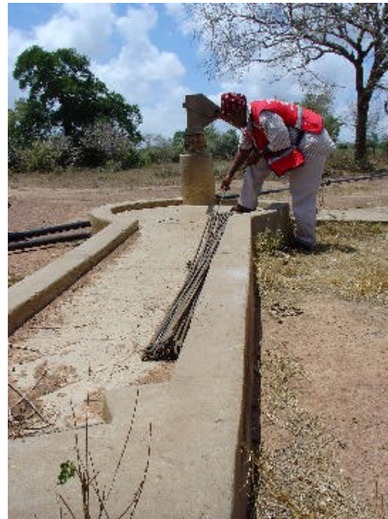
A broken and abandoned community water point.
