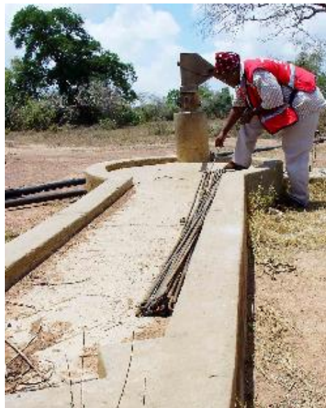
Rehabilitation of water points is a major component of this operation. Here, the Kenya Red Cross branch coordinator inspects a broken water pump in Kwale district.
