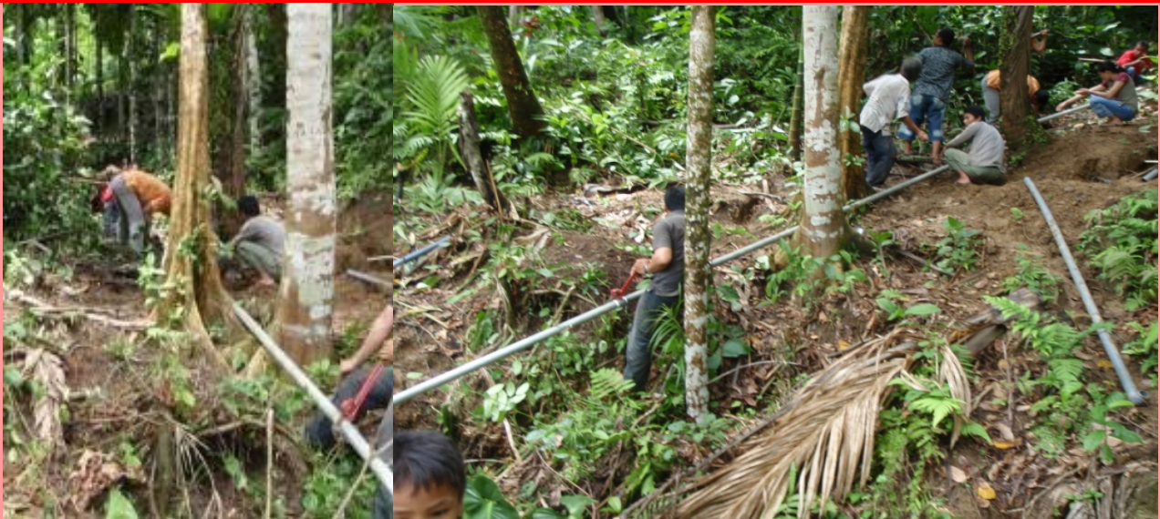
Villagers and International Federation's technicians lay piping through the jungle for Sisobaoho village. International Federation/Neil Hitchen
