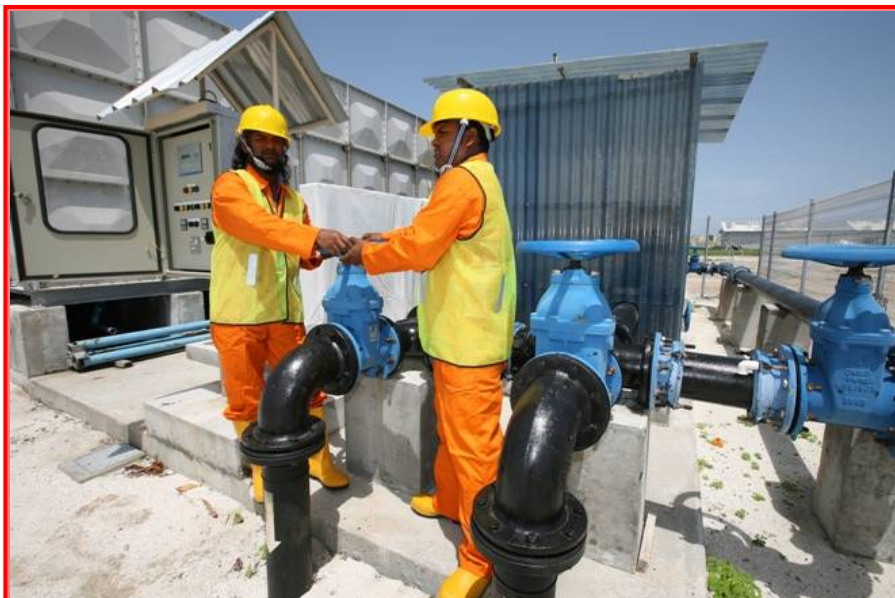
Alitho and Mohamed are two of the thirteen sewer operators who were trained during by the International Federation. In this picture, they are doing a routine check at the out-fall pump station, which pumps all the island's wastewater 200 m away from the reef into the deep sea. International Federation/Ahmed Zahid
