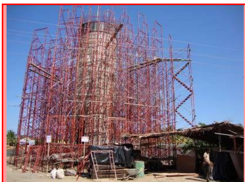
Construction of the Akkaraipattu Hospital Water distribution system and sewerage system. International Federation.
