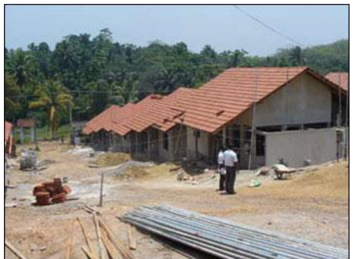
More than 2,000 houses are under construction on 74 sites across 11 districts in the county.
