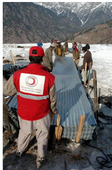
More than 127,000 sheets of corrugated galvanized iron were distributed in just nine weeks. (Photo: IFRC)
