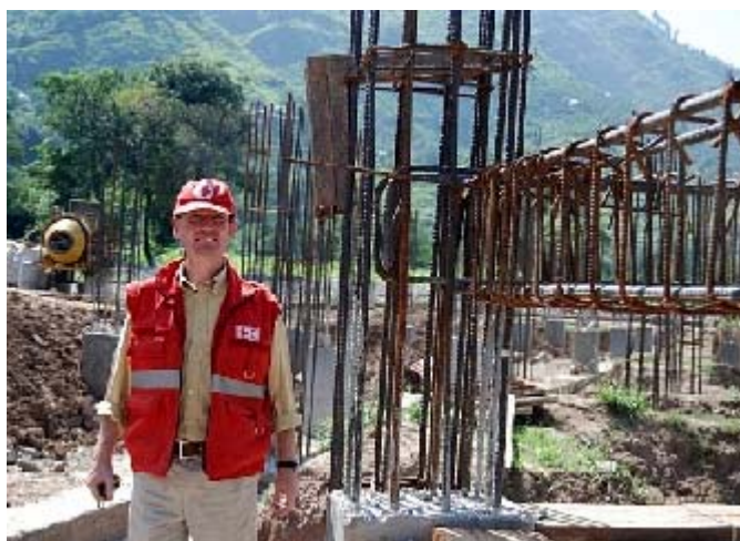
Construction work for a middle school for girls at Mera Bakot, Pakistan-administered Kashmir. (Photo: IFRC)
