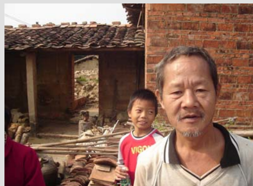
Mr. Zhong Zuxiao, 50 years old, stands in front of one of the houses destroyed by flooding in July. One of the main reasons the houses are destroyed is because they are built from unbaked mud bricks.
