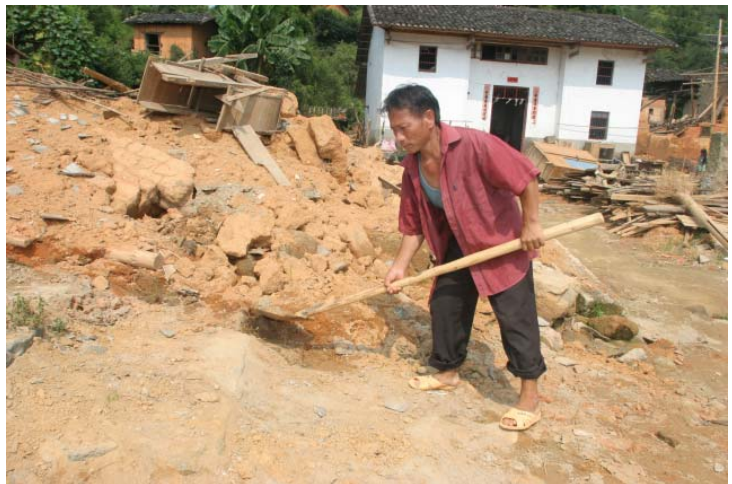
A villager clearing the debris caused by the typhoons.
