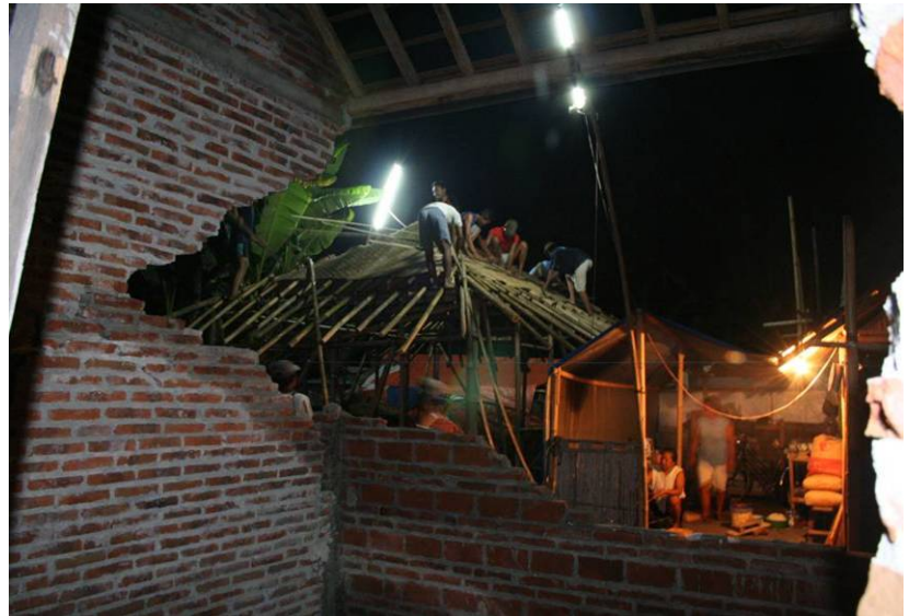
Communities work together at night to build the bamboo houses so they are able to work during the day in income generating activities.
