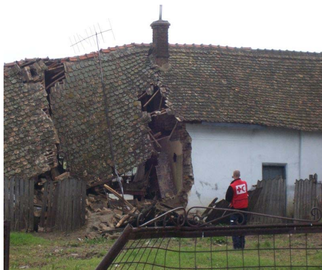
Floods that swept through the village in Rast have collapsed the brick structures of houses
