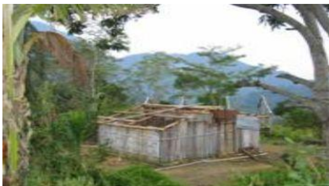
Strong winds stripped many houses of their roofs, exposing the poor structure of most houses in the affected areas.
