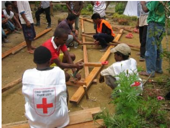
Communities were taught to build stronger roofs that would weather strong winds, keeping families safe in their homes during storms.
