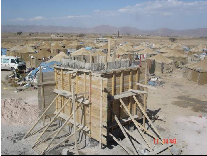
Concrete water tanks serve as a link between floods victims and better water supply
