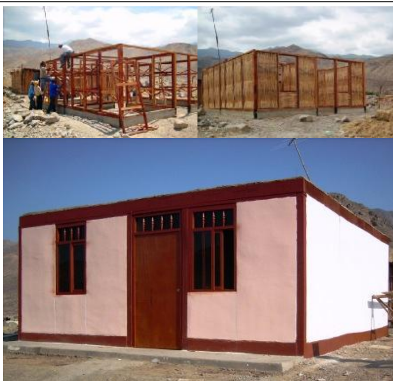
Model house built by CIDAP with the improved quincha technique in different stages of construction. International Federation / P. Caveró
