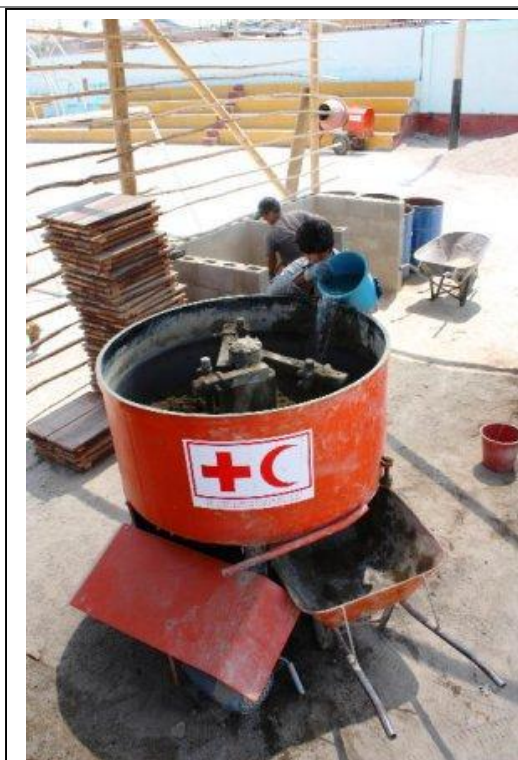
In San Clemente (Pisco), members of the community make compressed earth and cement bricks for the construction of their own houses. International Federation / J.Ormeño
