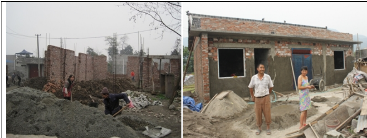
Despite a high level of completed housing reconstruction in urban areas, many families, like these two couples in Jiulong and Zundao Townships, are still reconstructing their homes in rural areas. Photos: Amanda West/ American Red Cross and Sho Huang/ International Federation
