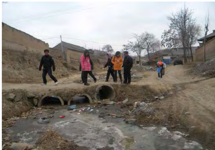
The county branch also inspected a collapsed riverbank and bridge in Wahuang Village, Qinan county, Gansu Tianshui prefecture as part of the VCA conducted. RCSC.
