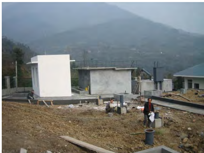
Sedimentation and filtration tanks at water treatment plant by the end of November. Photo: IFRC
