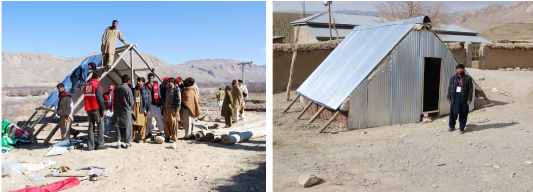
The PRCS/IFRC team working at a model shelter (left). A completed model shelter (right). Photo: International Federation.
