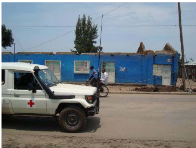
One of 1,982 houses in Gisenyi Town (Rubavu District) that was damaged by the extreme wind.
