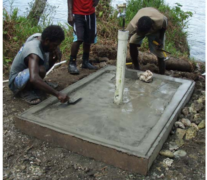
A group of Solomon Islands Red Cross volunteers fixing pipes for tap-stands in Kena, Kolombangara (International Federation).
