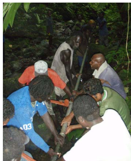
Community members and SIRCS volunteers working together to fix leakages on a PVC main pipe at Kuzii, Kolombangara Island (International Federation).
