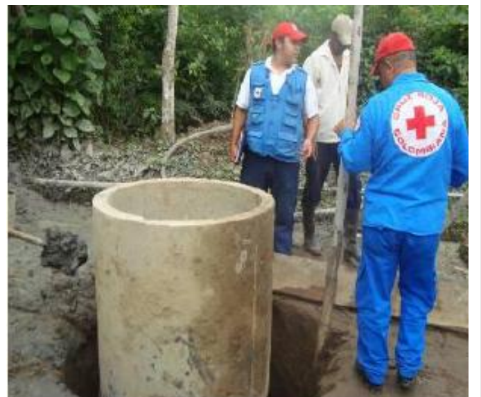
Construction of a water well with a capacity of 5,000 litres in Tumaco. Source: Colombian Red Cross Society
