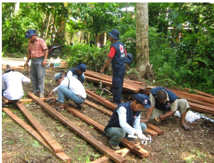
The t-shelter pilot project has begun in the the sub-district of Pariaman Utara in Padang Pariaman. Up to 37 PMI volunteers will build a total of 65 t-shelters in approximately ten days. Photo: Ony Purwitasari/ Spanish Red Cross.
