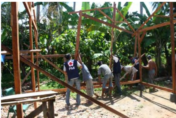
Construction of T-shelters in Kota Pariaman district continue, with 31 shelters successfully completed to date. Photo: Palang Merah Indonesia.
