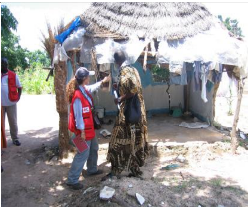
The FACT shelter delegate (Spanish Red Cross) assessing a seriously damaged dwelling in Kaolack.
