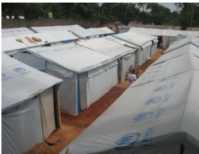
CAR Red Cross volunteers constructed shelters for the beneficiaries with support from UNHCR/IFRC
