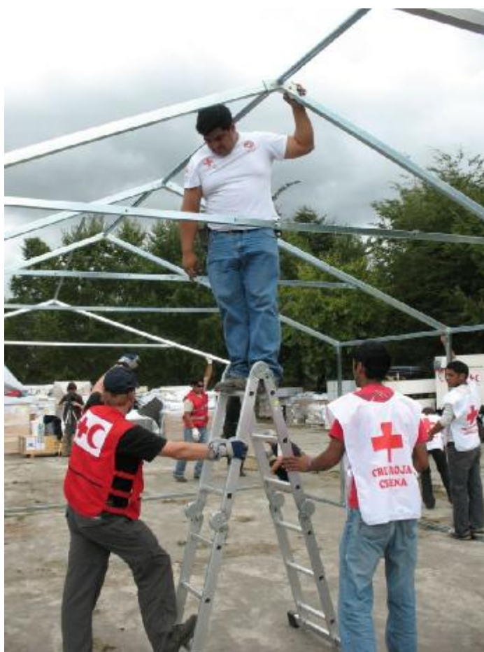
Chilean Red Cross volunteers and Finnish/Norwegian delegates installed the surgical hospital in Pitrufquén in the region of La Araucanía. Source: Norwegian Red Cross
