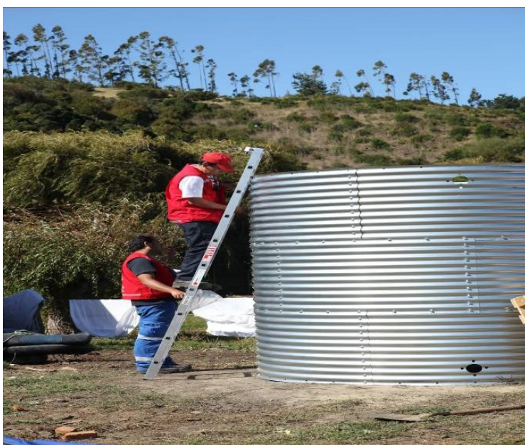
Chilean Red Cross volunteers installed water tanks in Tubul. Photo source: International Federation
