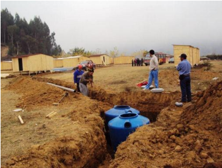
Sanitation modules in process of installation in the region of Bio Bio. Photo: German Red Cross.
