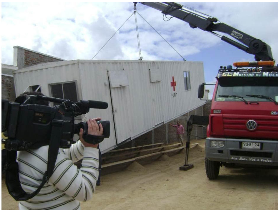
Delivery and installation of the field branch donated by Shell Chile to replace the collapsed branch constitution. Source: Chilean Red Cross.
