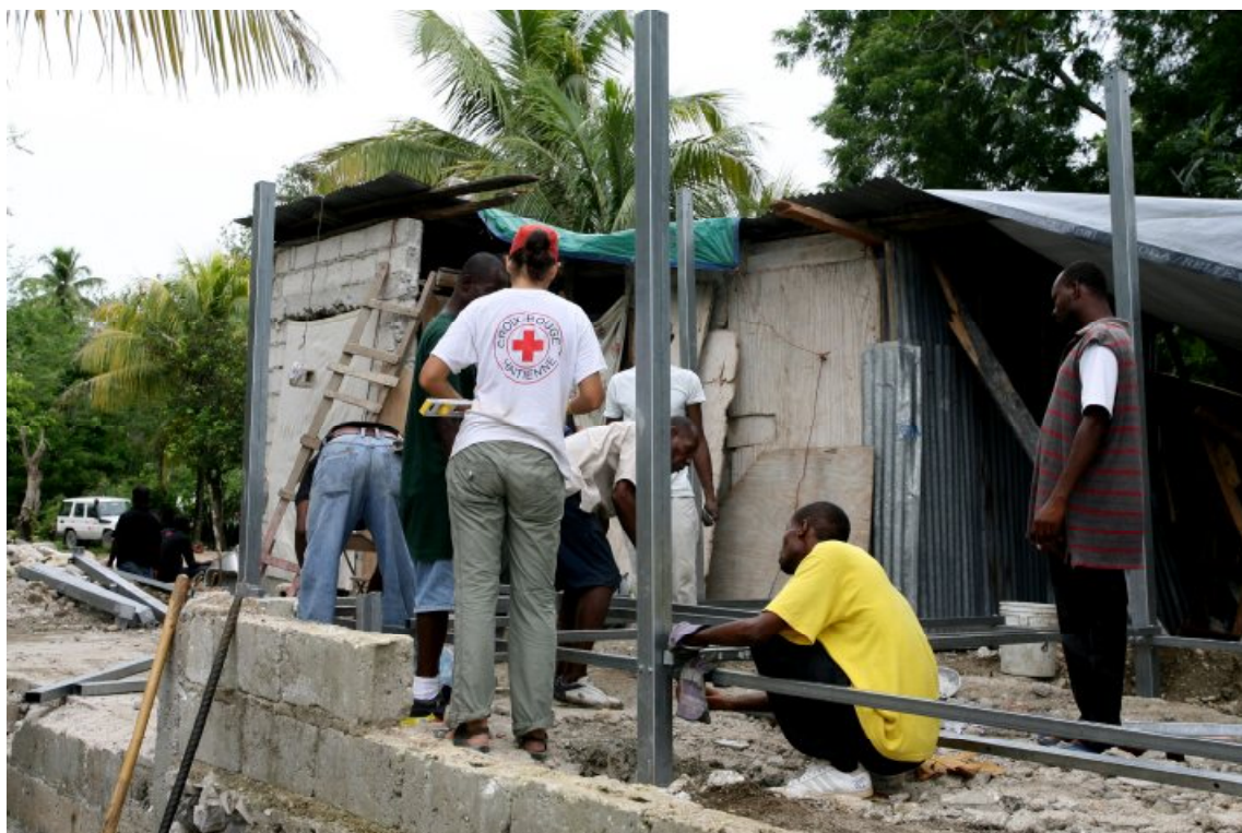
The Spanish Red Cross construction team busily engaged with the construction of their first transitional shelter in Leogane. Source: José Manuel Jimenez/IFRC
