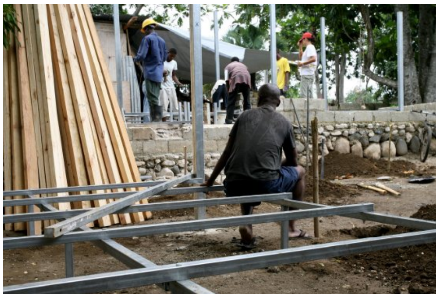
The Haitian Red Cross Society volunteers and the Spanish Red Cross construction team busily have started the construction of their first transitional shelter in Leogane. Source: José Manuel Jimenez/IFRC
