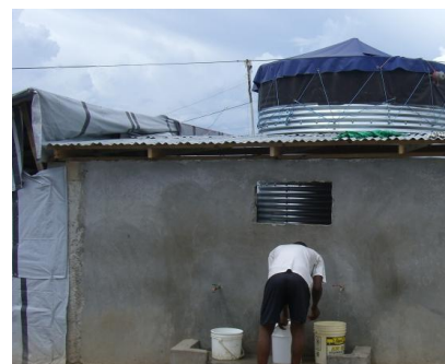
IFRC completed construction of this water reservoir, enabling private vendors to provide water to camp residents Source: IFRC
