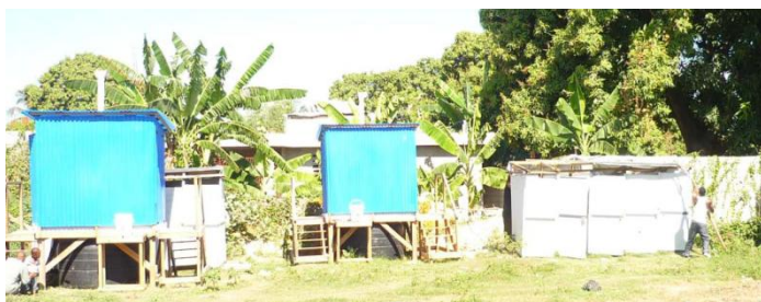
Tank latrines and showers installed at a camp Source: IFRC
