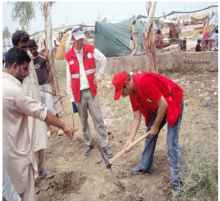
Water and sanitation disaster response team in Larkana is busy in constructing latrines. To date, 43 latrines have been constructed in Larkana. Photo: WSDRT IFRC
