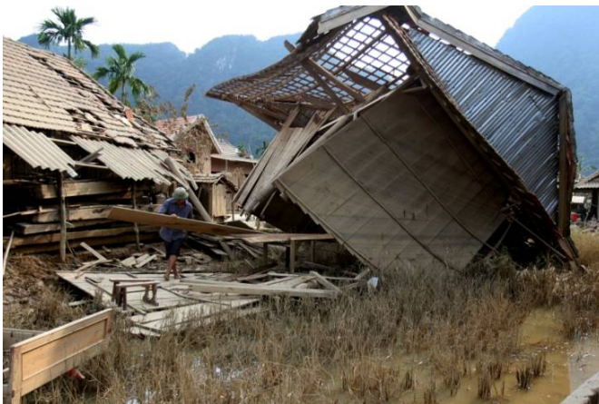
9 October 2010: Floodwaters washed away foundations causing houses to collapse in the Tan Hoa commune, Minh Hoa district, in Quang Binh province. (Photo: Tran Quang Tuan, VNRC)
