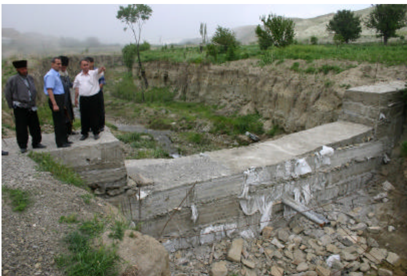
Landslide trap in Karaul village in Baharden
