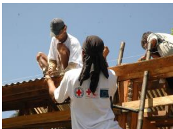
Promoting increased typhoon-resistant traditional shelter construction practices in the Philippines (International Federation)
