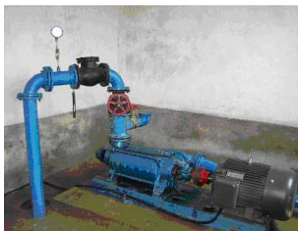
Interior of Red Cross installed WatSan pumping station
