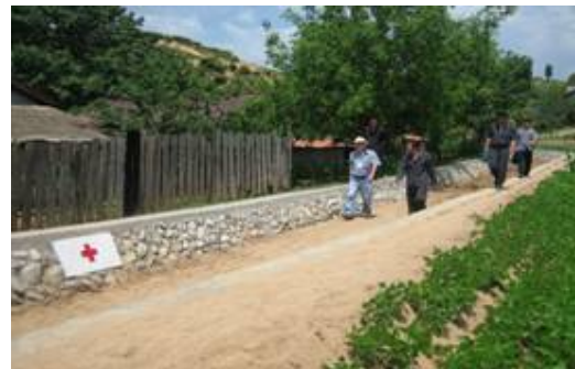
Inspection of newly installed water channels in Inda ri, Yungan county (S. Hamyong).
