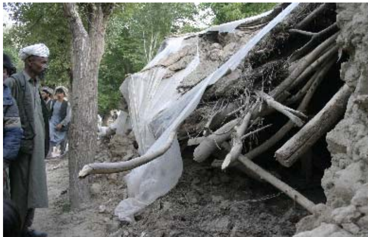
Villagers look at a collapsed building caused by the spring floods in Faryab district, Mazar. (Photo by ICRC)
