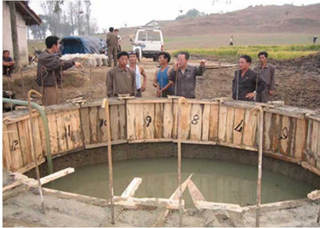
Field monitoring of the construction of a water source by DPRK Red Cross water and sanitation technician in Ryongsong-ri, Ryongchon county, North Pyongan Province.
