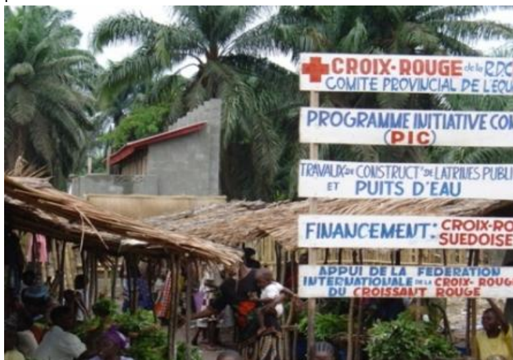
Construction of public latrines at a market in Mbandaka – Equateur Province, DRC
