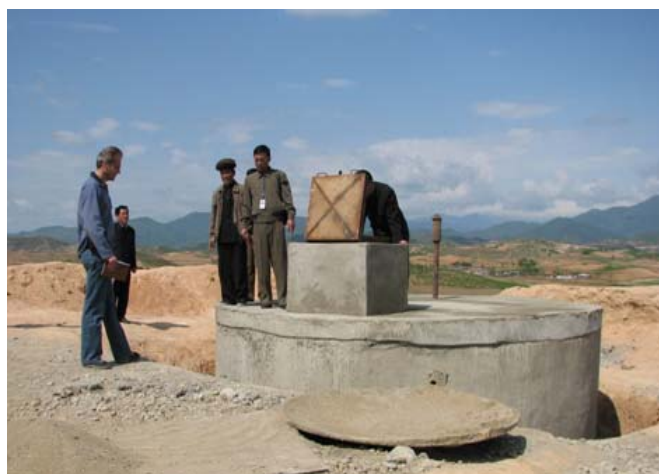
A newly constructed reservoir tank in Jaeon-ri, Hamju county, South Hamgyong Province, 14 May, 2008. International Federation.
